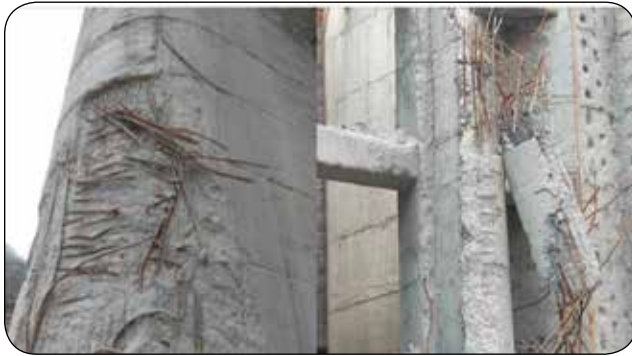
Damage on Barrage Pier and Intake structure
