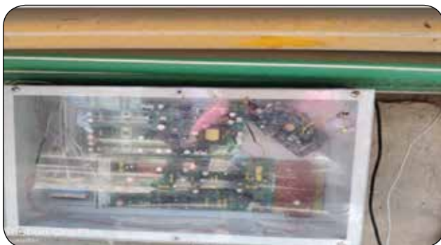
Prototype Broken Rail Detection System At ShaheenBagh
