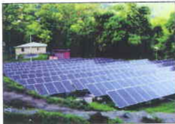
60 KWp Off-grid Solar PV Power Plant installed at Office of Sashatru Seema Bal (SSB), Sapri, Himachal Pradesh
